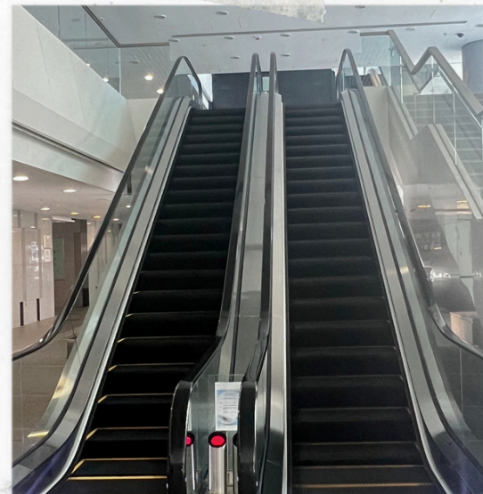
Figure 5-4: Optimising the energy saving mode of escalator in the Office Building of CAD Headquarters
