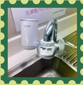
Figure 5-18: Faucet with higher water-saving efficiency in the pantries
