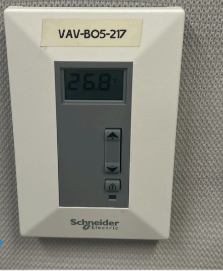
Figure 5-1: Air conditioning setting of at least 25.5°C
