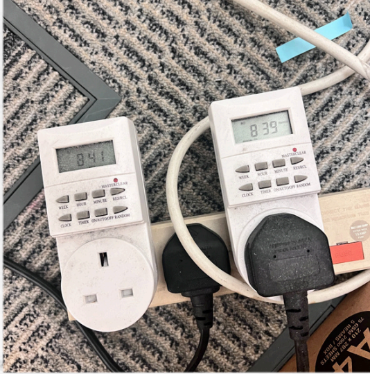
Figure 5-6: Installing energy-saving timer devices in printers and photocopiers during non-office hours
