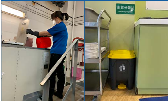
Figure 5-14: Food waste decomposition system in CAD Headquarters and Food Waste Collection area in Canteen
